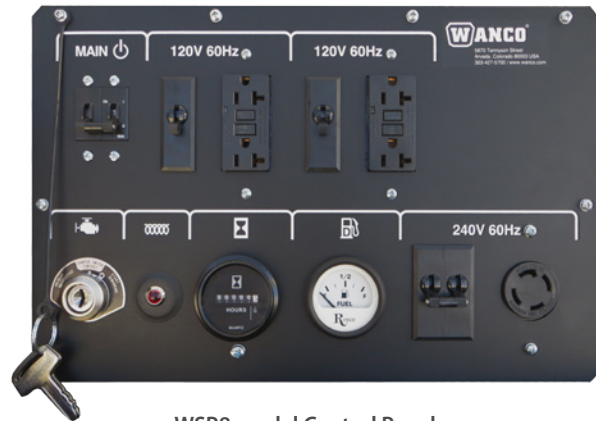
WSP8 model Control Panel (Located inside)
